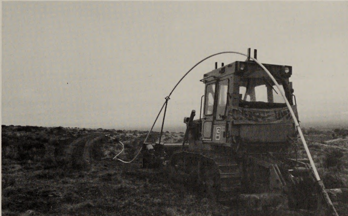
The pre-coupled pipe is fed through a series of guides and rollers mounted on dozer and cab of tractor. Pipe finally enters ground through a 3-1/2- inch tube shaped into a gentle arc. Depth capability is governed by ripper tooth assembly. This particular line is going in at a depth of approximately three feet. Although not shown in this photo, a twenty-foot piece of anchor chain is dragged in a "U" pattern behind pipe-layer to pull soil berm back into the furrow.
